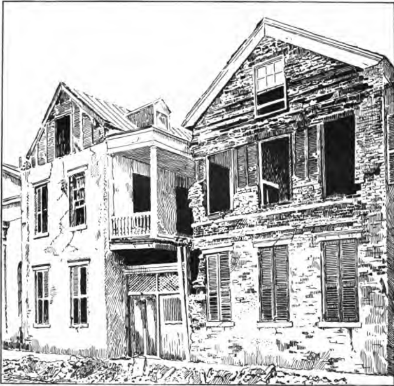
FIG. 197. VIEW OF PART OF CHARLESTON, S.C., WRECKED BY THE EARTHQUAKE OF AUGUST, 1886
